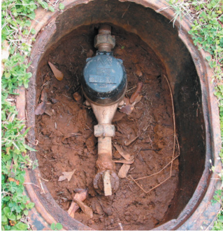
Proper Residential Meter Installation in Pit Setting
